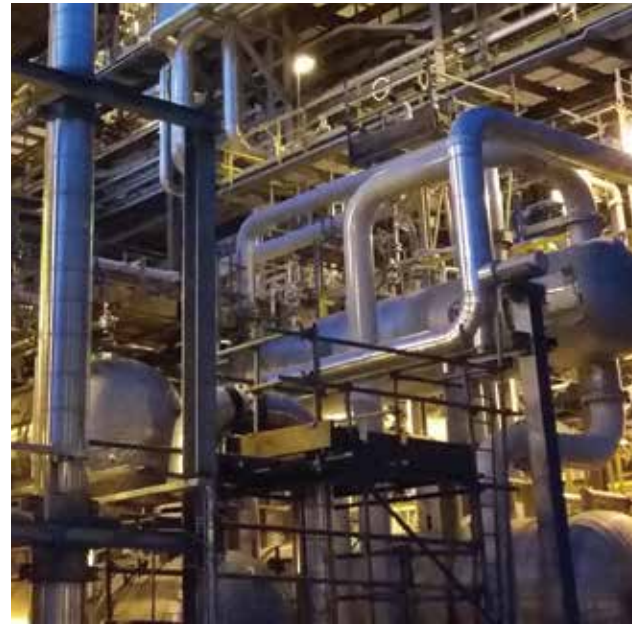
Industrial & Process Cooling Refrigeration
